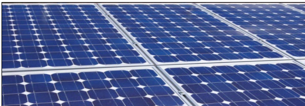
Figure 11. Module Spacing Gaps
